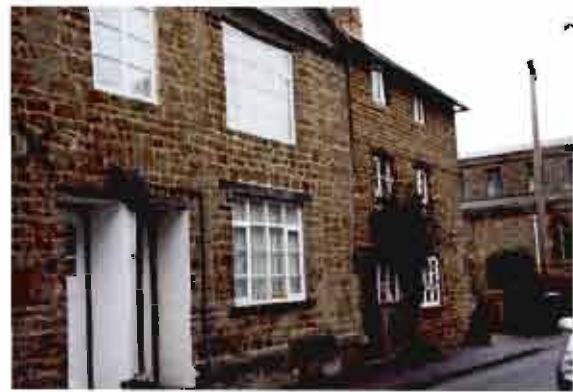
Example of black painted timber lintels and black painted structural cross bracing
